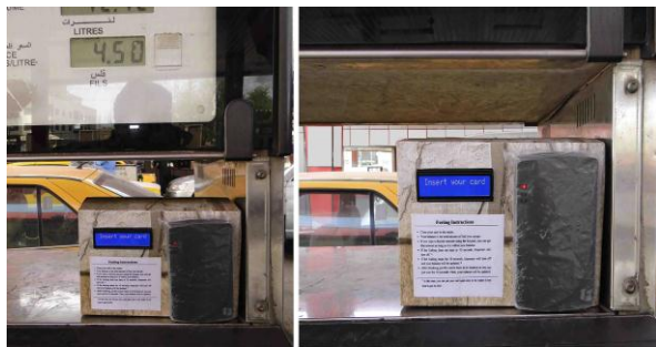
Figure 10. Hardware module attached to dispenser at a station
