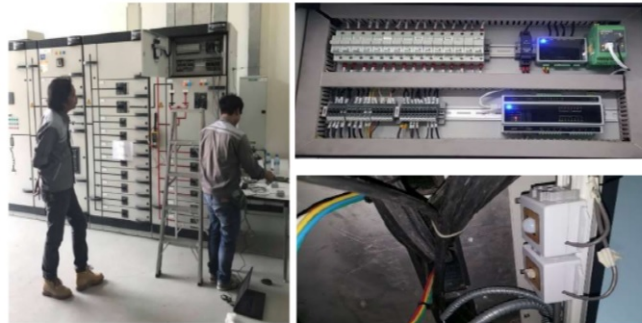
Figure 4. The installation of IoT in an electrical switchboard
