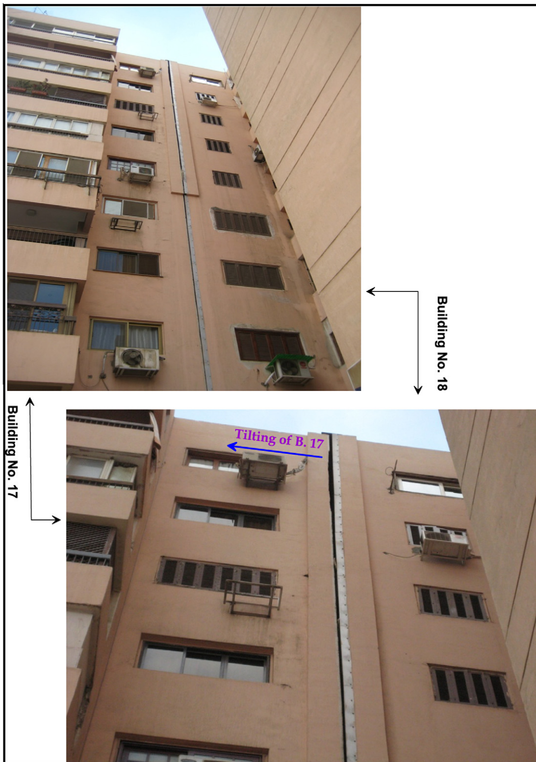
Figure 3 Tilting of Building No. 17 relative to Building No. 18.
