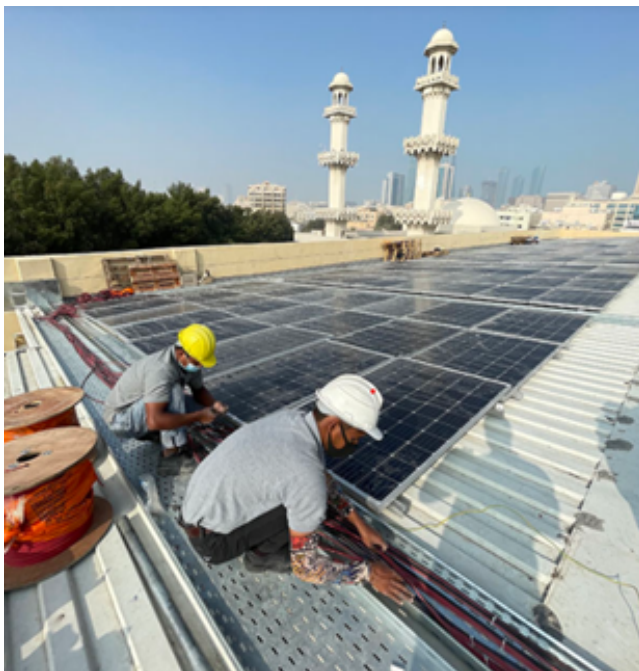
Figure 4. Solar Photovoltaic Installation
