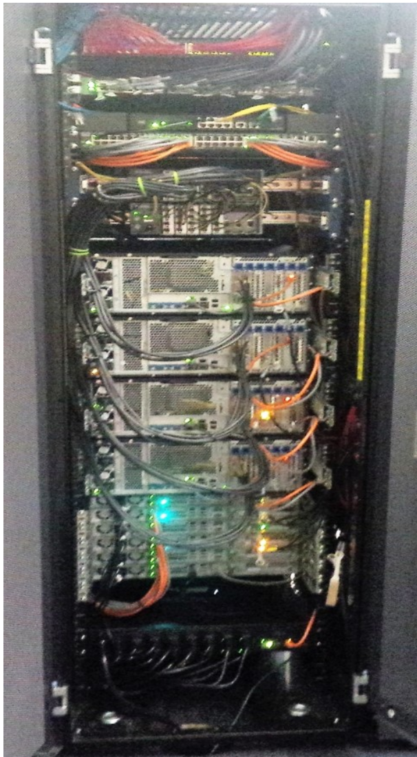
Figure 5. Four node Ivy Bridge cluster with instrumentation
